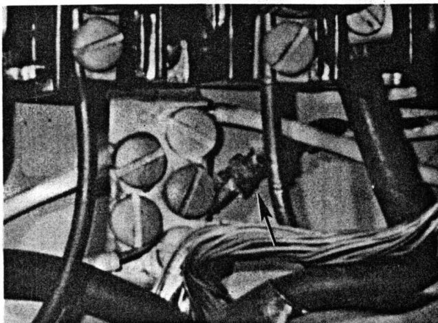
FIGURE 11 - WIRE TERMINALS ON ALUMINUM BUSBAR
